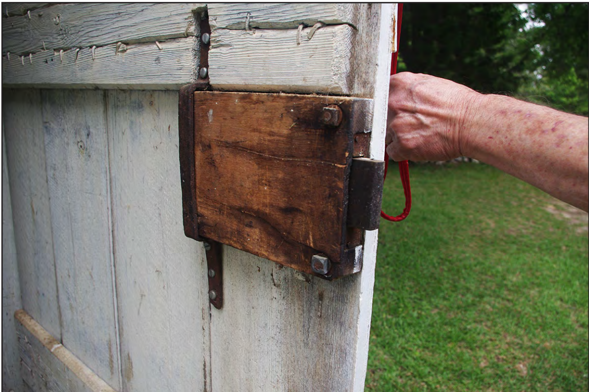
PLATE 84: Detail of Door and Original Boxed Lock on Smokehouse, Elliot-Terry-Mossor Farm (RH0297), Rockingham, North Carolina
