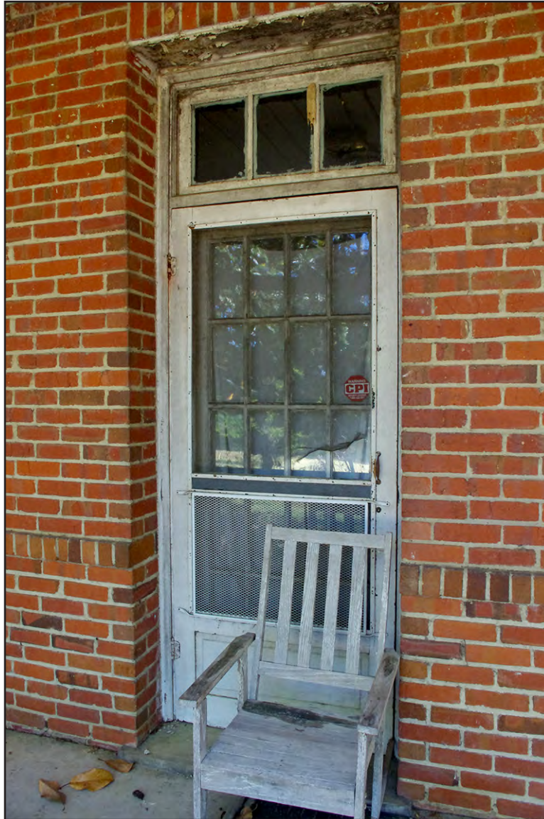
PLATE 13: Glenwood Rest Home (County Home) (RH0667), Main Entrance Detail on South Elevation, Rockingham, North Carolina
