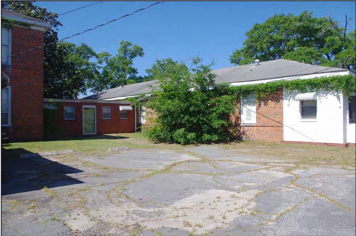
PLATE 20: Glenwood Rest Home (County Home) (RH0667), North Elevation of Western Hyphen and East Elevation of Western Wing, Rockingham, North Carolina
