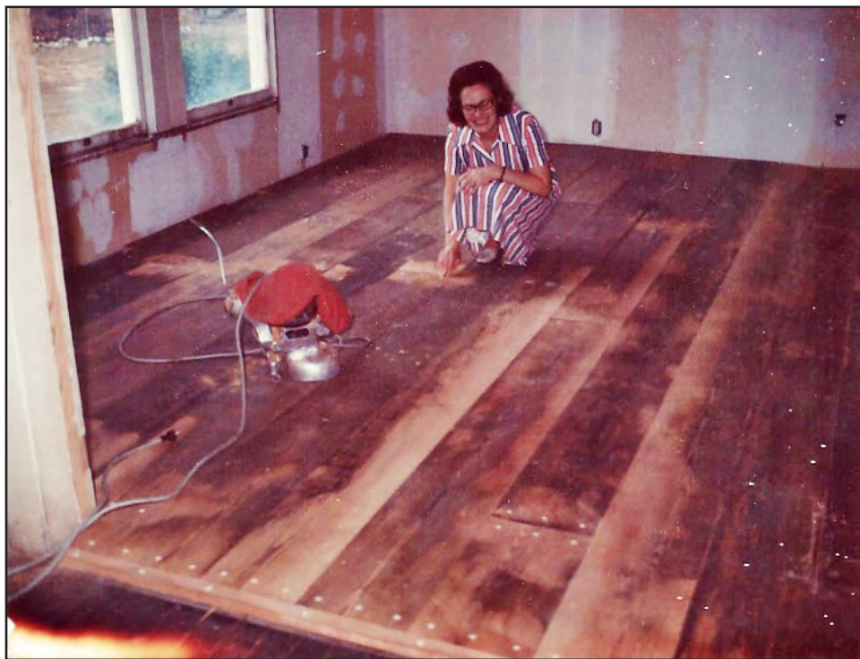
PLATE 100: Mabel Mossor Sanding Cherry Wide-plank "Pegged" Floors Installed During 1970 renovation, Dining Room, Facing East, Elliot-Terry-Mossor House (RH0297), Rockingham, North Carolina (Courtesy of Jim Mossor)
