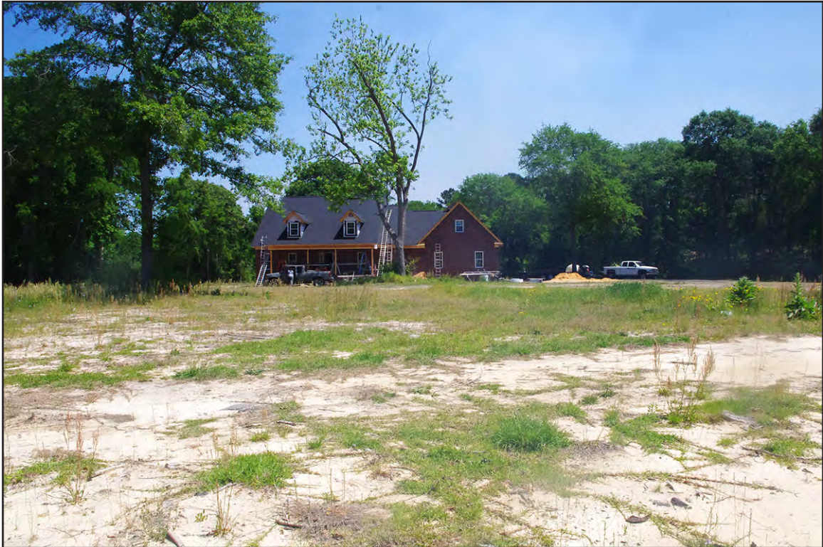
PLATE 66: Sam Covington House (RH0364) Property, Showing Old House Demolished with New House Being Constructed in Its Place, Looking North, Rockingham, North Carolina
