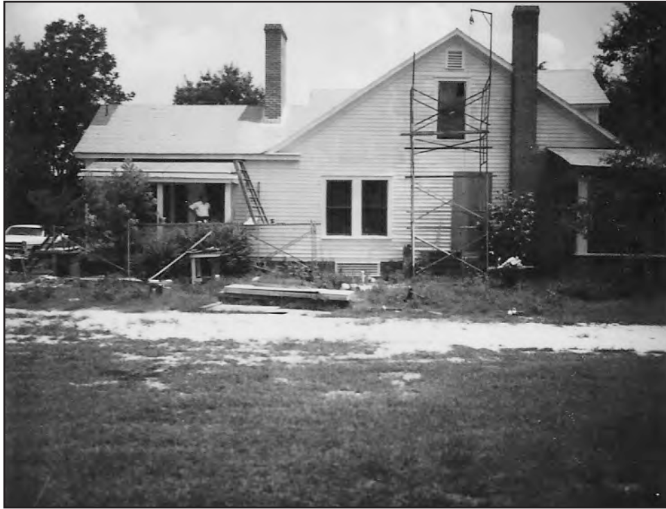
PLATE 103: South Elevation of Elliot-Terry-Mossor House (RH0297) During 1970 Renovation, Rockingham, North Carolina (Courtesy of Jim Mossor)
