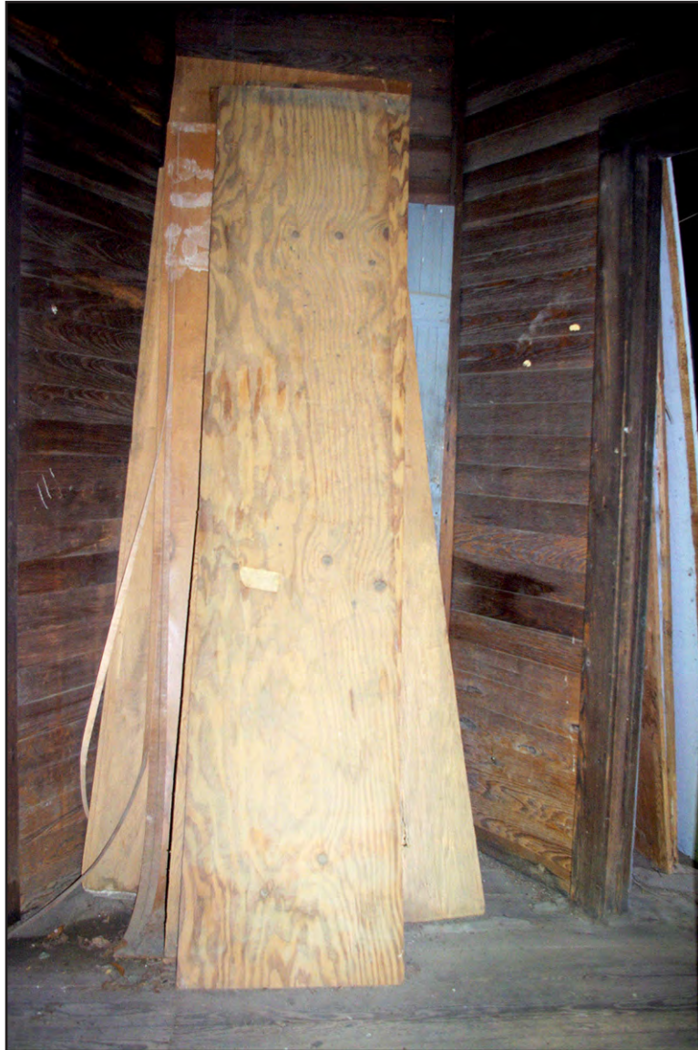
PLATE 95: Detail of Interior Trapezoidal Entryway of Dwelling No. 2, Elliot-Terry-Mossor Farm (RH0297), Rockingham, North Carolina
