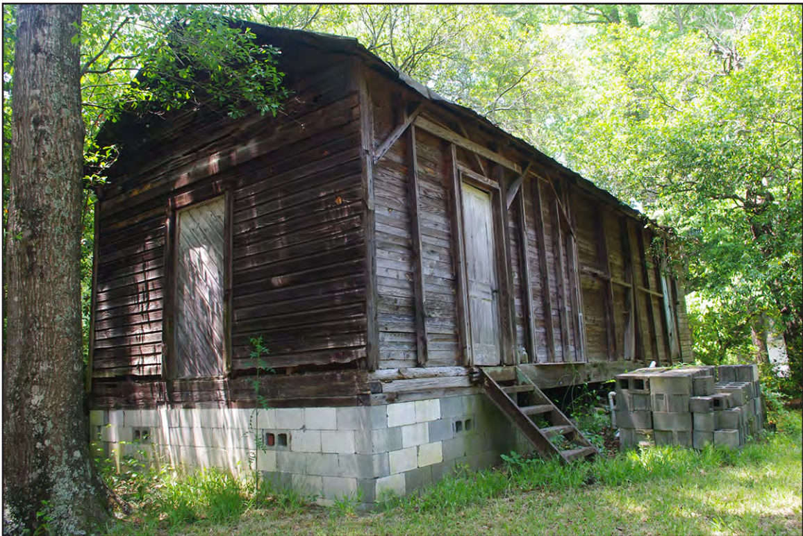
PLATE 81: Terry Store, Oblique View of East and North Elevations, Elliot-Terry-Mossor Farm (RH0297), Rockingham, North Carolina
