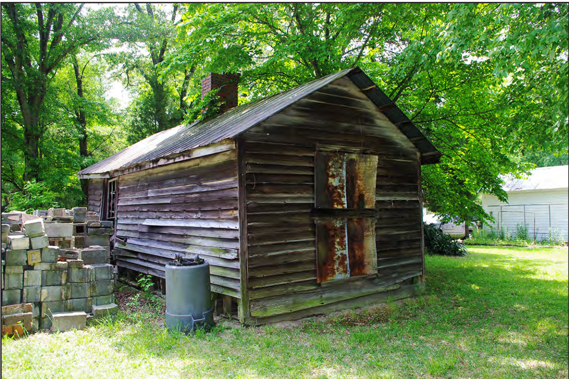
PLATE 90: Cook/Help House, Oblique View of West and North Elevations, Elliot-Terry-Mossor Farm (RH0297), Rockingham, North Carolina
